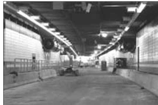
Vast tunnel project uses Vibro-Acoustics silencers on jet fans as a key part of the emergency ventilation system.
